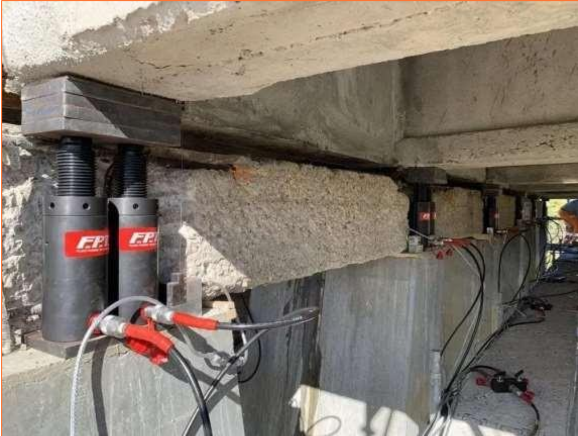
Hydraulic Jacks and Pumps
